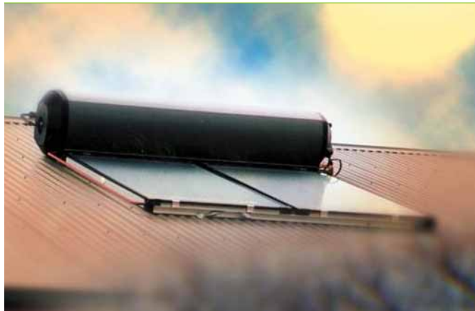
A typical solar water heater.
