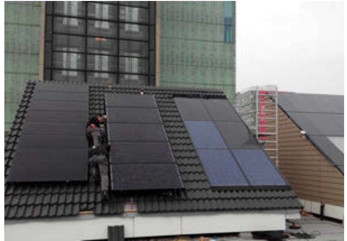
▲ BIPV project SolarBeat. Left PVT panels, middle PV panels and right 3 PVT panels and 3 solar thermal collectors.
